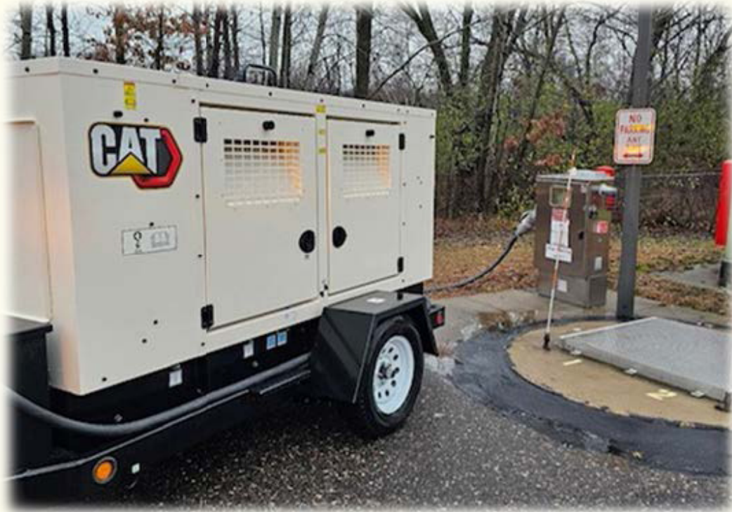
Photo: Generator successfully tested at one of our lift stations, demonstrating full operational capability.
