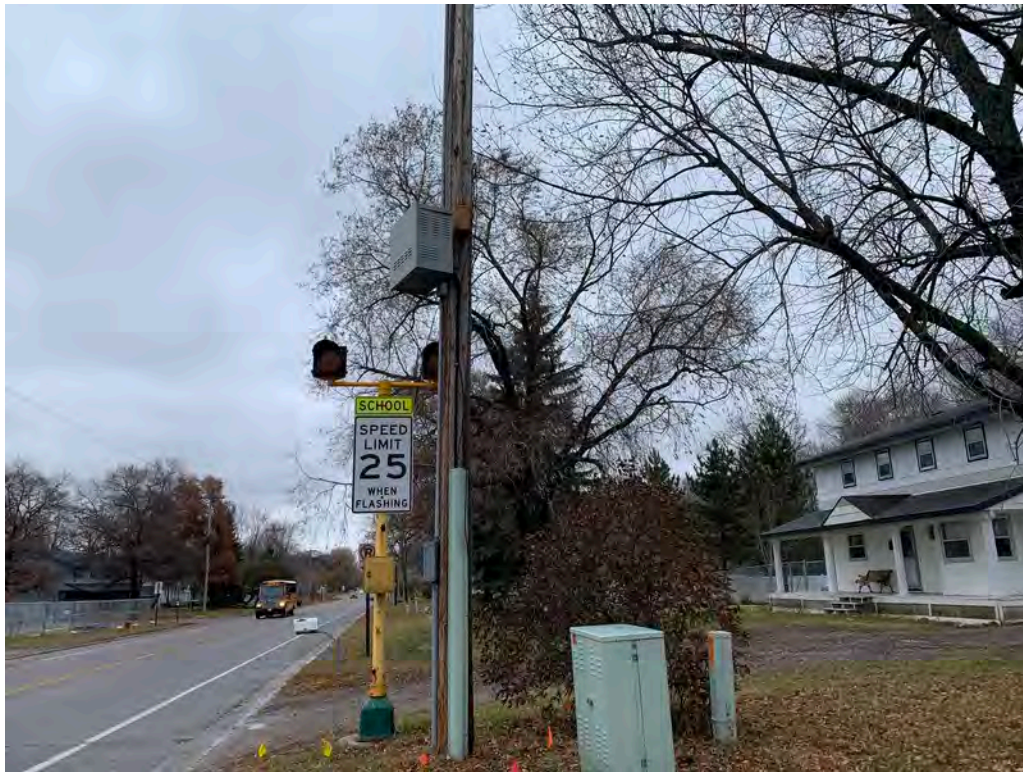
Photograph 5 - View of transformer located in the northwest corner of the Property.
